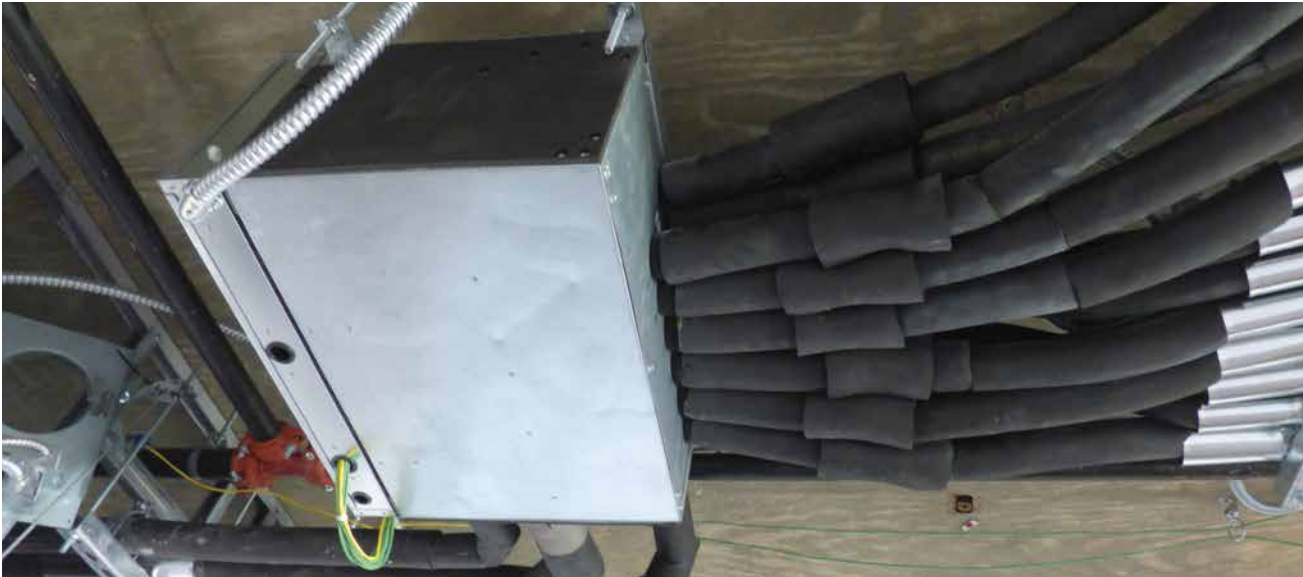
Insulation from Daikin Units to Branch Controller
